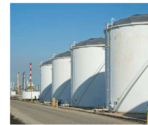
Oil Storage Tank
