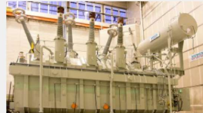
System-interconnecting transformer in high-voltage substations
