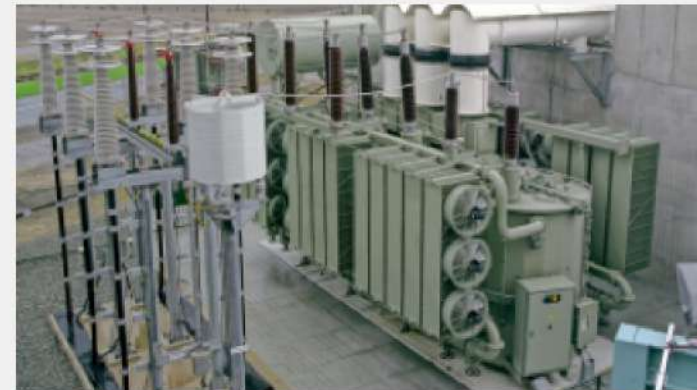
Unit auxiliary transformer
