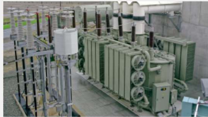
Unit auxiliary transformer
