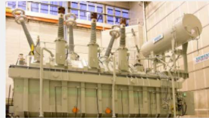
System-interconnecting transformer in high-voltage substations
